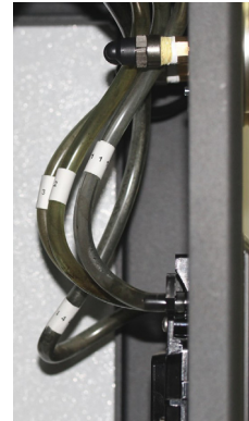
Bad tube routing
