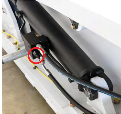
Relief valve located next to hoses on cylinder manifold
