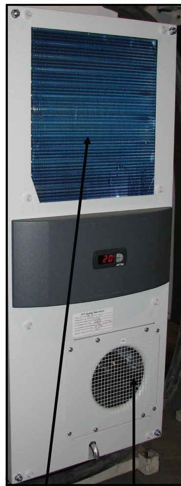
Blow out the Fan and Compressor Fins.
