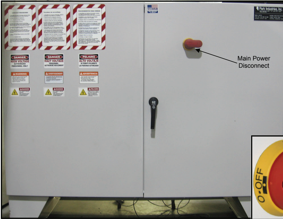
Electrical Cabinet, Doors Closed
