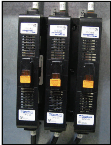
AC Line Fuses
