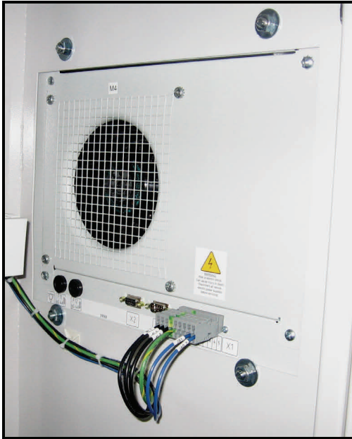
Inside Electrical Cabinet (Back Side of Unit)
